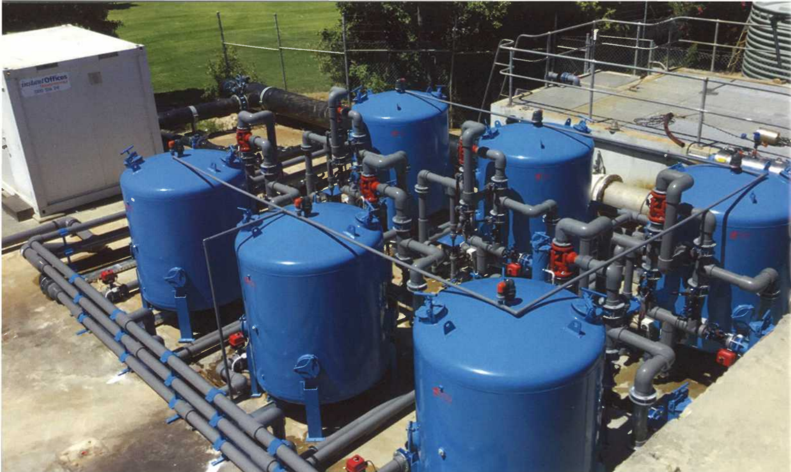
Above: Ozone Reserve filtration system
