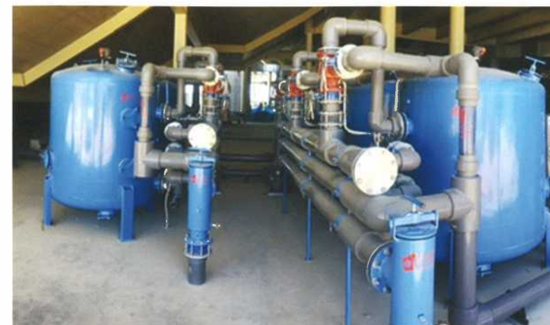
Above: Bore Water iron filtration system installed at Optus Stadium. Photo: Elliotts Irrigation
